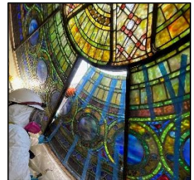
The Nzilani worker is removing the first panel from the rose window.
